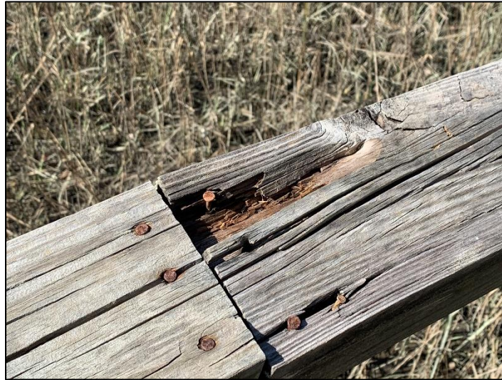
Figure 3.1. Severely Split or Deteriorated Top Railing
