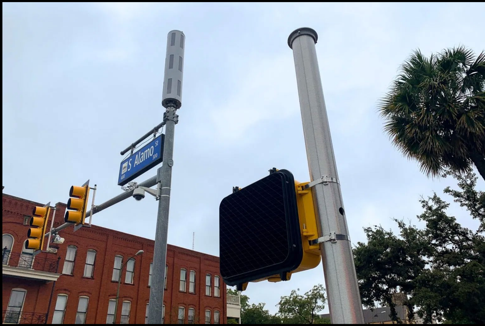
Traffic light with antenna attached. (San Antonio, TX)
