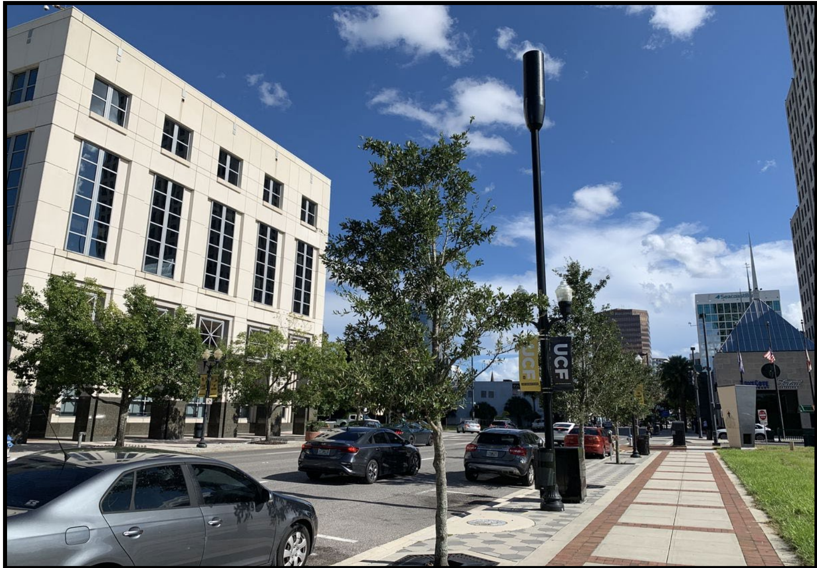
Light post with attached small cell antenna and associated ground equipment cabinet. (Orlando, FL)
