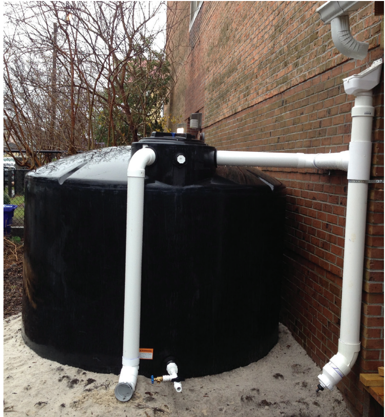
Figure 4.6-1. Example Cistern Application (Photo: Marty Morganello)
