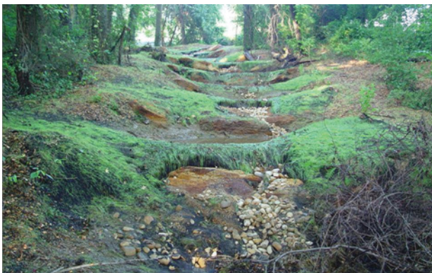
Figure 4.8-1e. Regenerative Stormwater Conveyance (Photo: Biohabitats, Inc.)
