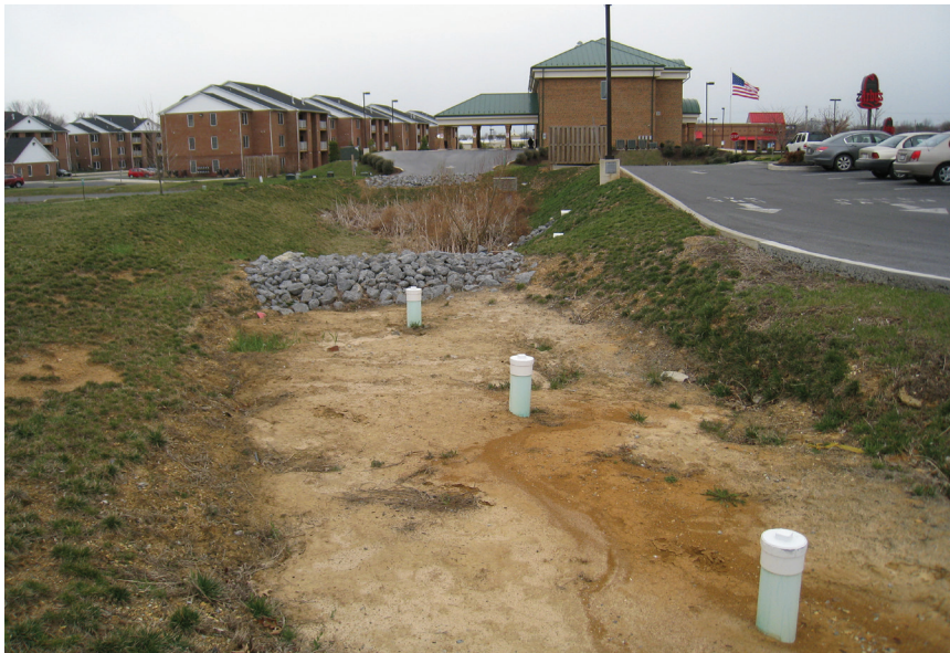
Figure 4.4-8. Infiltration Sand Filter Example (Photo: CWP)
