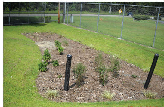
Figure 5.2-2. Bioretention cell at Loris Recycling Center (Photo: Horry County Stormwater Management)
