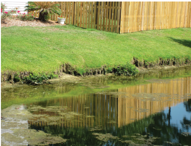
Figure 5.1-2. Bank erosion prior to restoration treatment (Photo: Diane Smith)
