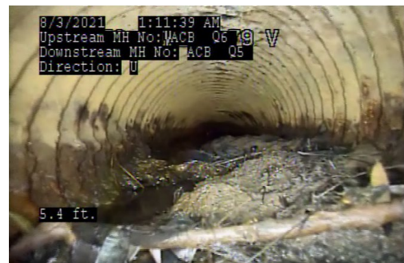
Figure 1 – Blockage in 18" CMP
