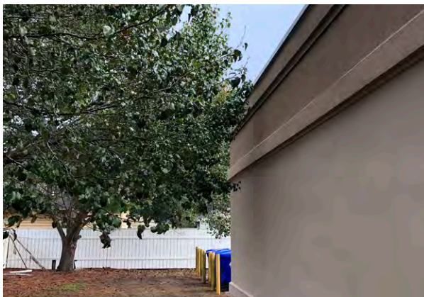
Trees are brushing up against the building
