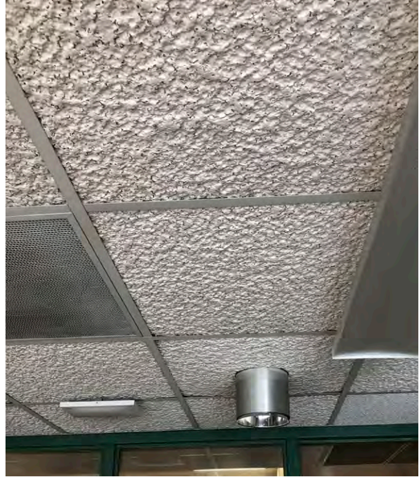
Ceiling grid is damaged in some locations and tiles are sagging
