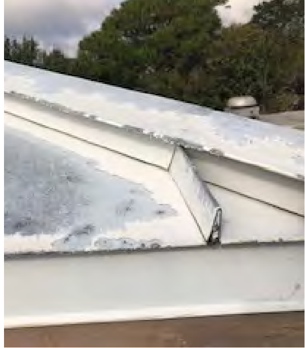
Damaged paint on standing seam roof
