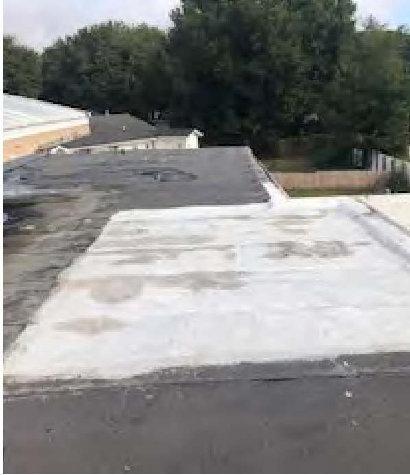
Membrane roof is patched in some areas
