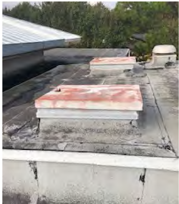
Mechanical space access hatch
