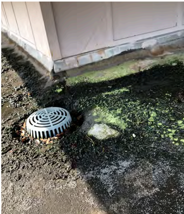
Example of debris / ponding surrounding roof drains
