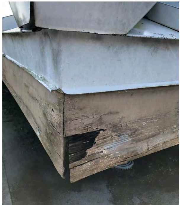
Rotten fascia board
