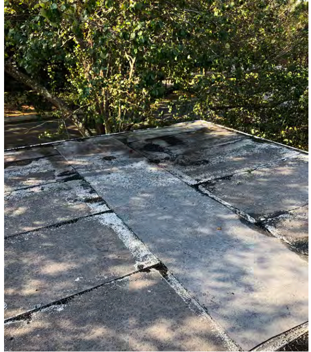
Membrane roof is patched in some areas
