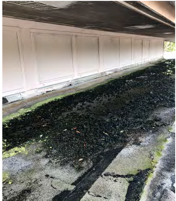
Clerestory windows are boarded up and painted - alligatoring and debris is present throughout
