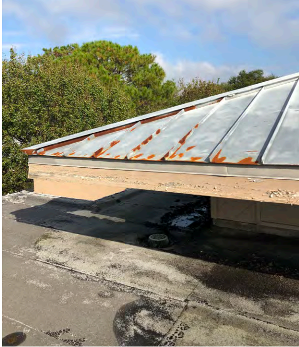
Standing seam roof is rusting
