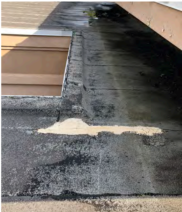
Membrane roof blisters
