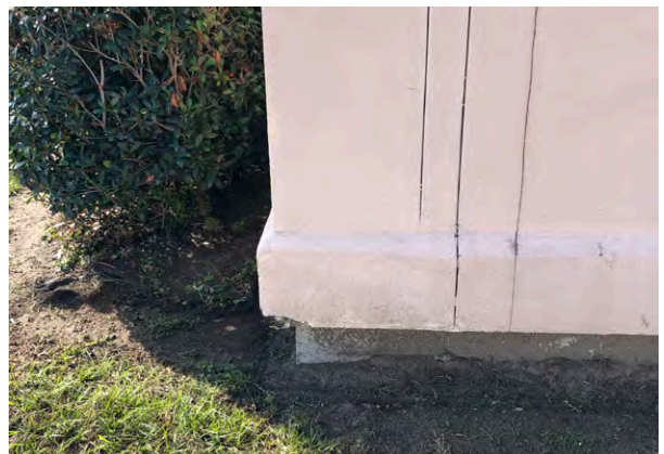
Damaged EIFS at several locations along the perimeter
