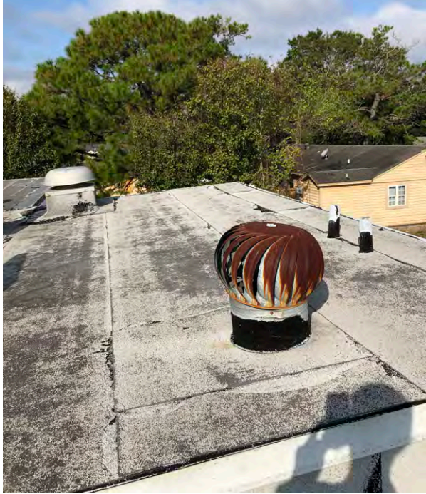
Fan is not functional
