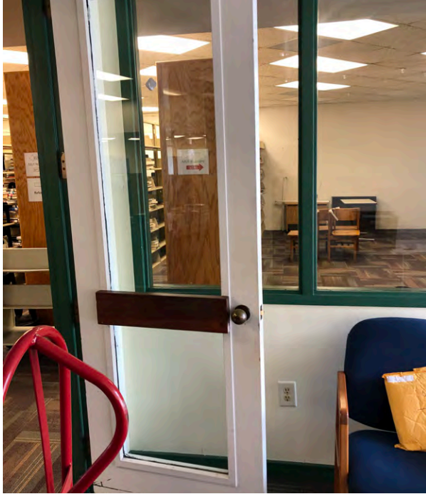
Damaged door leaf at the office
