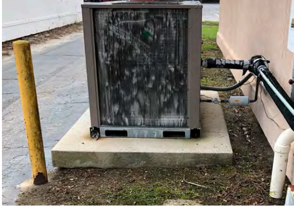
Damaged fins need re-combing and the curb is eroding
