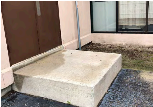
Loading dock step needs additional step for access
