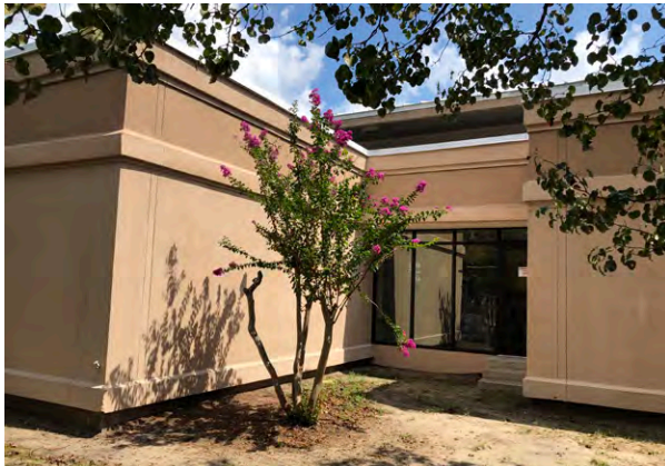
West Facade - Rear Entrance. Stair requires a handrail.
