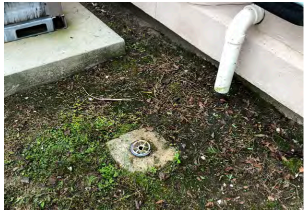
Clean-out is damaged
