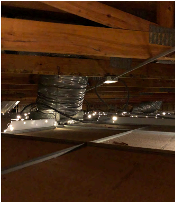
Ceiling grid, lights, etc. are not seismically installed - plenum spaces in the three open rooms is limited
