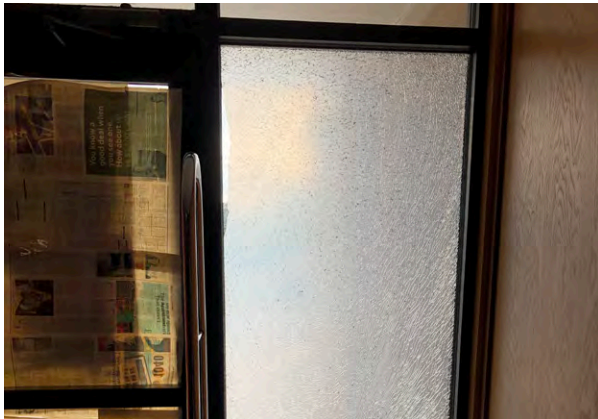
A pane of tempered glazing is shattered at the entrance
