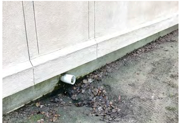
Erosion around the roof drains
