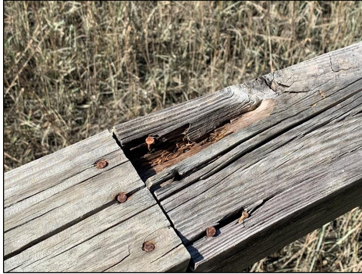
Figure 3.1. Severely Split or Deteriorated Top Railing
