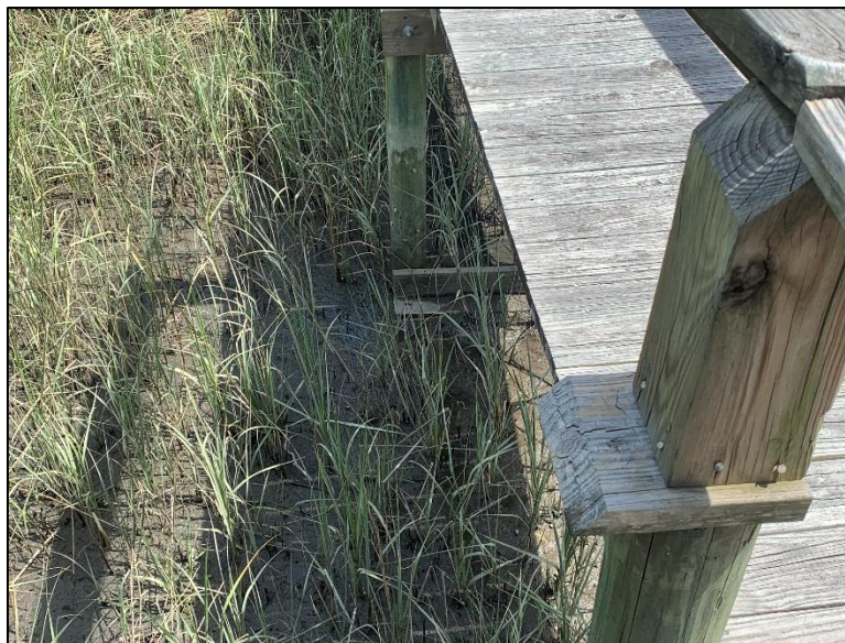
Figure 3.5. Lumber attached to Piles at Marsh Line
