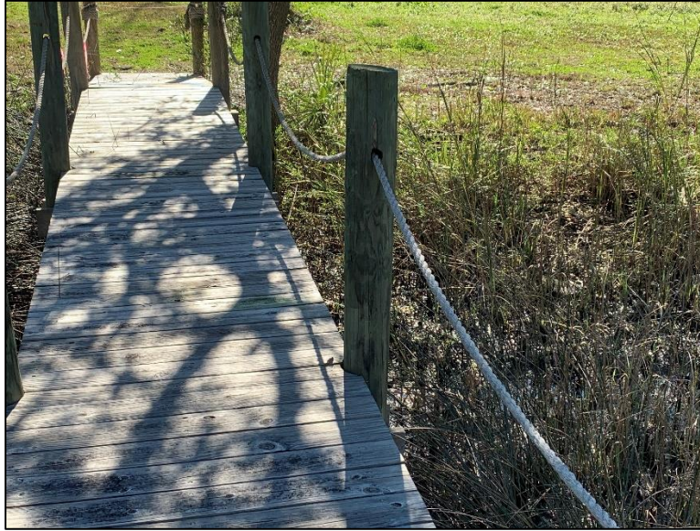
Figure 2.2. Rope Railing installed in Holes Through Timber Piles
