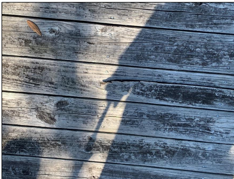
Figure 3.4. Decking that is Split and Showing Signs of Deterioration
