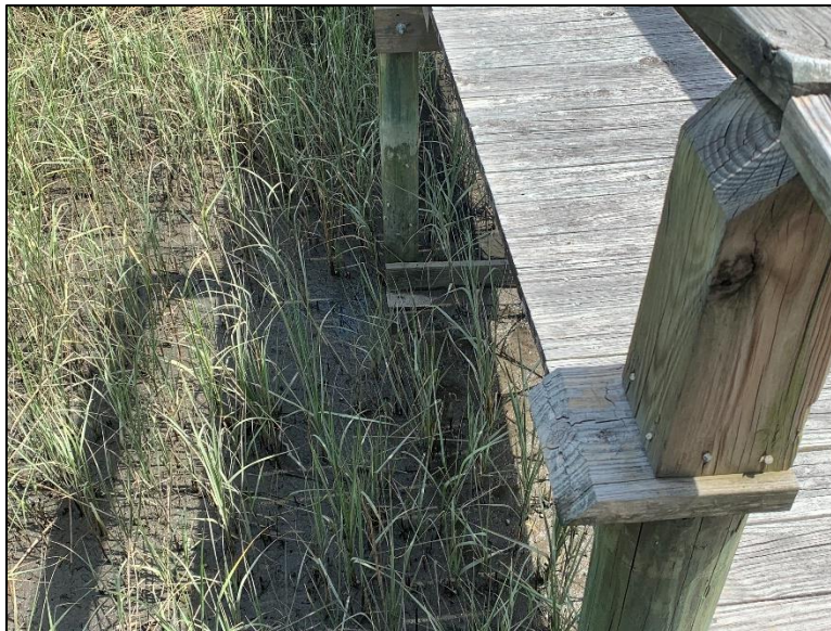
Figure 3.5. Lumber attached to Piles at Marsh Line
