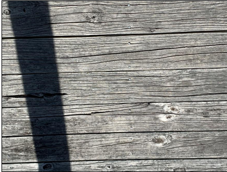
Figure 3.3 Decking that is Split and Showing Signs of Deterioration
