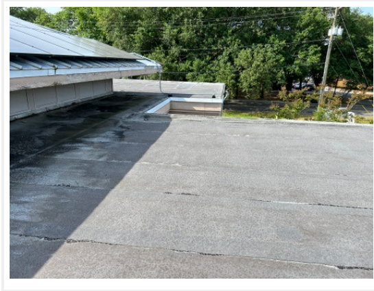
Photo 2 Overview of roof. Roof surfacing (minerals) have completely worn off. Roof has passed it's useful life and is deteriorating rapidly.
